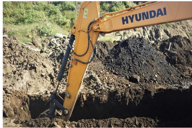
Photo 2. Excavation in order to reach the soil layer underlying the cast iron sand waste
